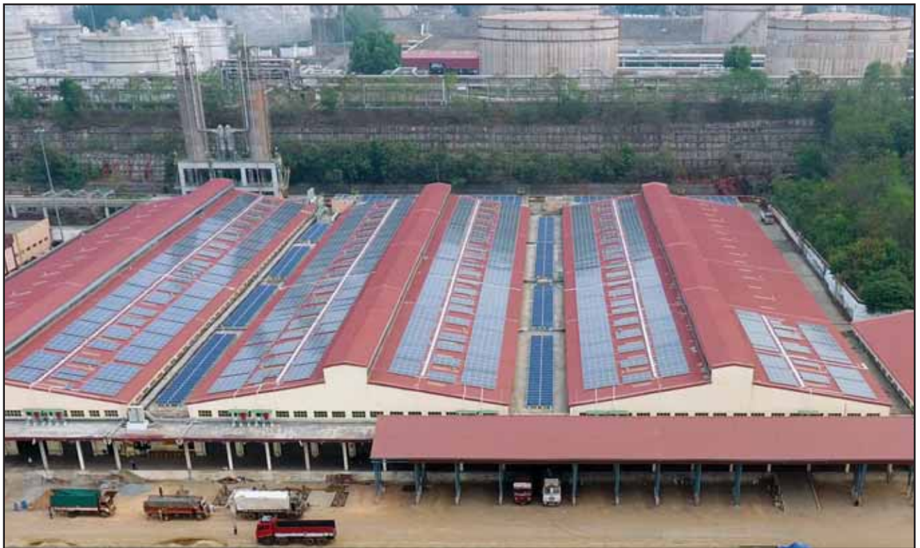
SOLAR POWER PLANT AT MRPL REFINERY
