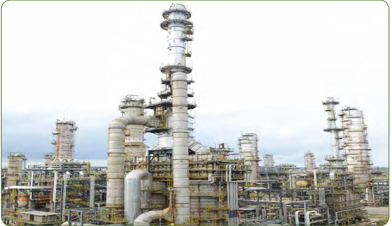
OMPL Process Units
