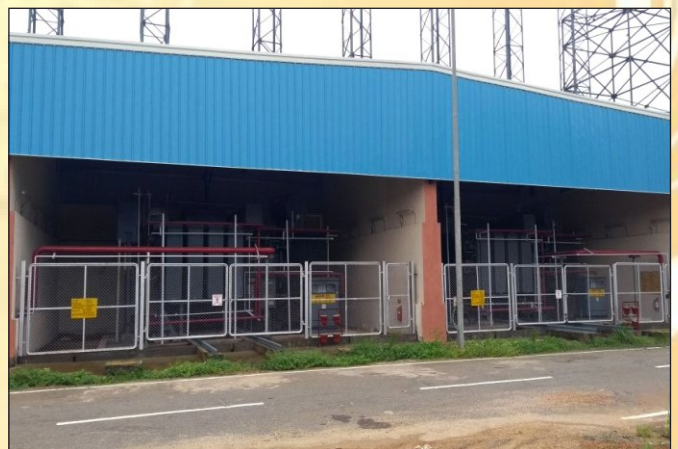
MRPL – OMPL Power interconnection transformer
