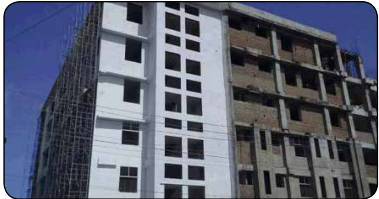
Lady Goschen Hospital, Mangalore – 5 story block from MRPL “AROGYA SAMRAKSHAN”, CSR initiative, work in progress.
